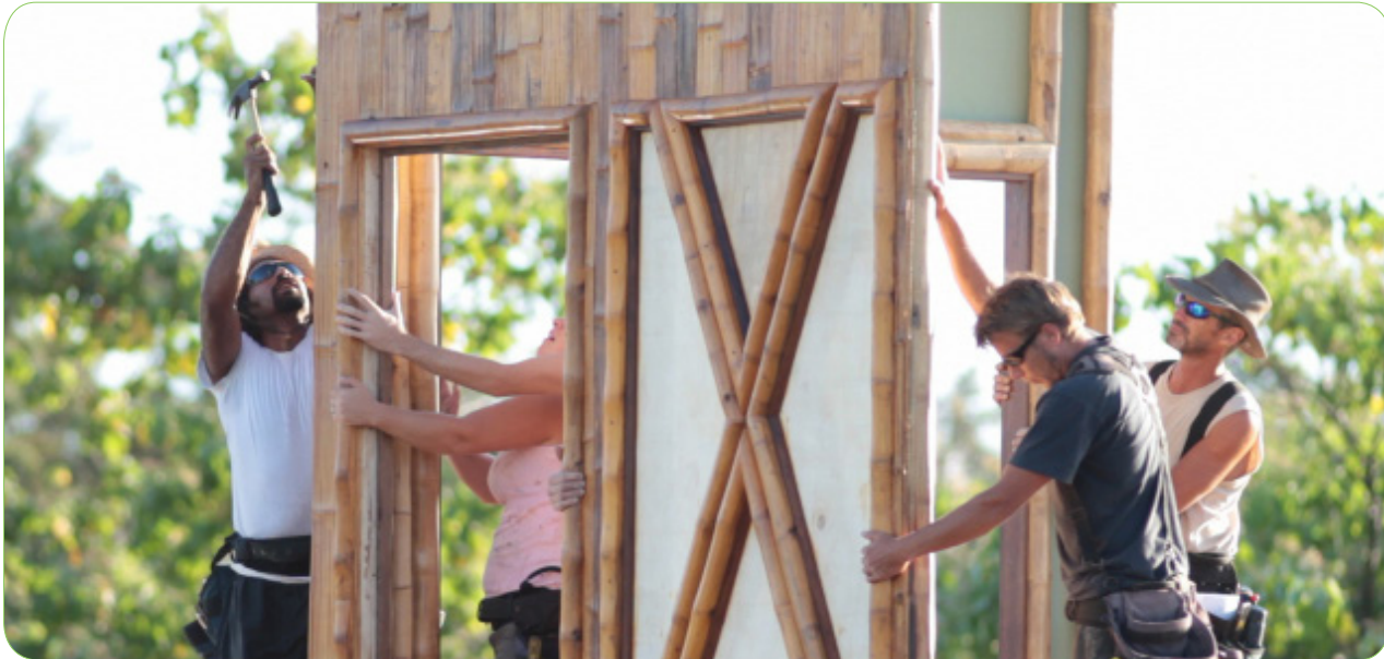
Contractors assembling the Bamboo Living exterior wall panels of a Signature Home Package.
